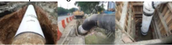
Langat 2 Water Treatment Plant and Water Reticulation System in Selangor / Kuala Lumpur Developer : Pengurusan Aset Air Berhad
