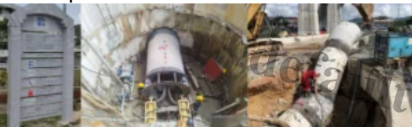
Langat 2 Water Treatment Plant and Water Reticulation System in Selangor / Kuala Lumpur Developer : Pengurusan Aset Air Berhad
